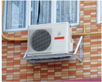
Supporting frame for an air-conditioning unit
