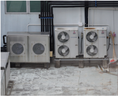
Supporting structure for an air-conditioning unit
