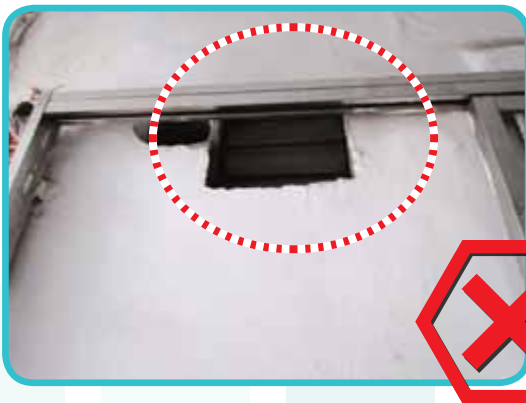
Ventilation opening is formed on the wall between the “subdivided unit” and the exit staircase/smoke lobby
