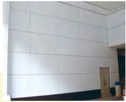
Panel fixed by metal dowels and fixings onto a wall inside a building
