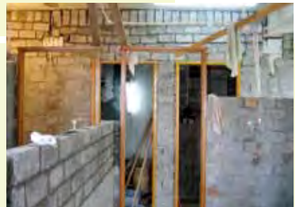
Erection of non-load bearing block wall, thickening of floor slab by laying solid screeding, or erection or alteration of aboveground drain in a flat
