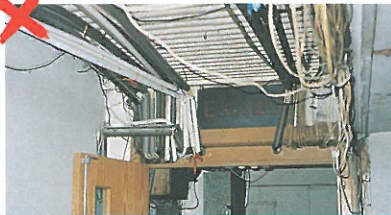
Services within staircase enclosure without proper protection
