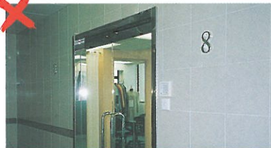
Door of inadequate fire resistance opens onto common corridor
