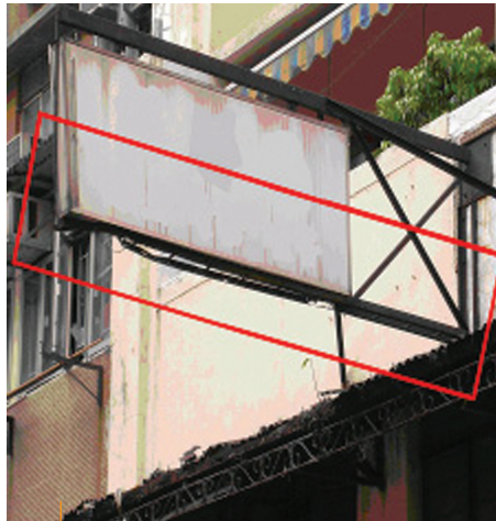
Signboards abandoned by moved away shops
