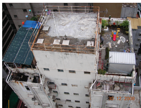
Unauthorised rooftop structures
