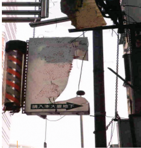
Corroded and tilted supporting metal frames
