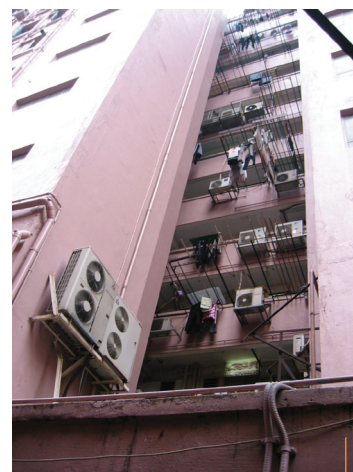
Supporting frames of A/C units on external wall
