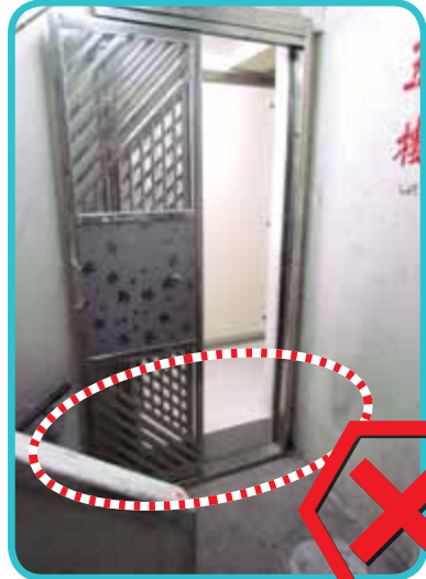
Excessive thickening of floor slab by laying solid screeding
