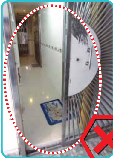
Exit staircase/smoke lobby is directly accessible from corridor of the “subdivided units” due to removal of the fire rated door at the original flat entrance
