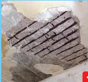
Spalling concrete/ exposed reinforcement
