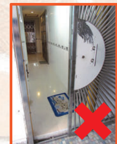
Existing fire rated doors removed or replaced by doors not meeting the required fire resistance rating
