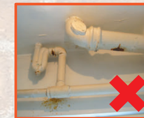
Water leakage in the additional and altered drain pipes
