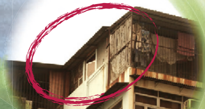
Remove any unauthorised building works
