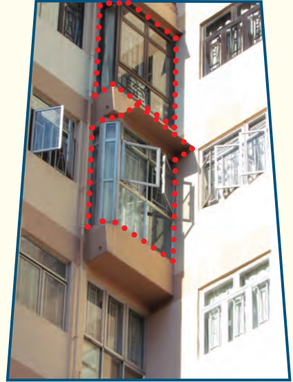
Window enclosure on approved planter
