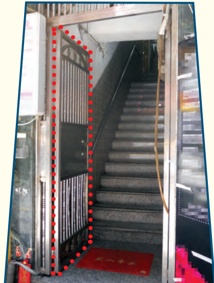
Metal gate obstructing the means of escape
