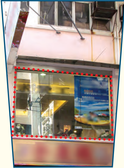
Large glass panels which do not comply with regulations
