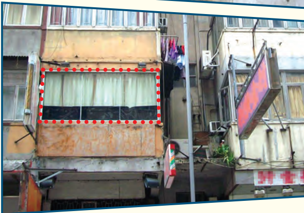
Enclosed balcony which does not comply with regulations
