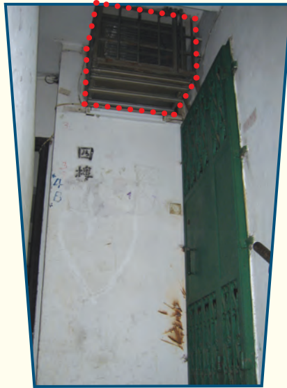
Opening formed in the staircase enclosure wall
