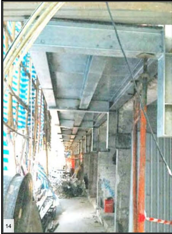
Corridor slabs were demolished and replaced by new structural steel decks (Source: Hong Kong Youth Hostels Association UNESCO Report)
