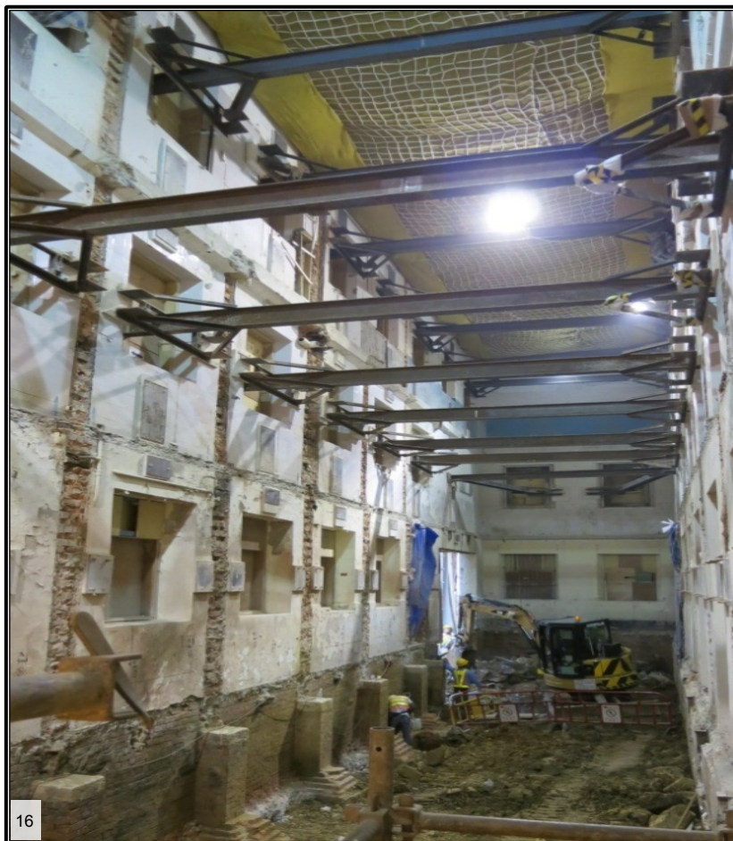
Temporary steel structures installed to provide lateral restraint to the retained facades during construction (Source: Arup)
