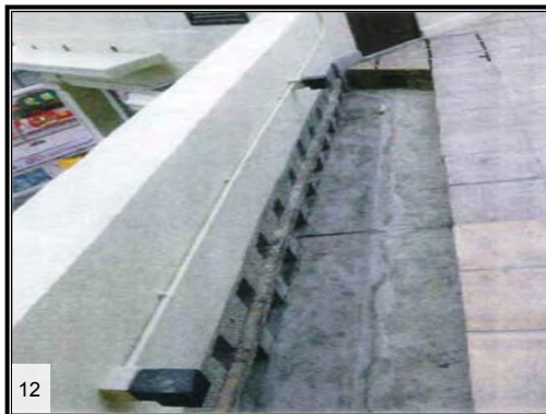
Canton tiles with insulation layer removed along the parapet walls
