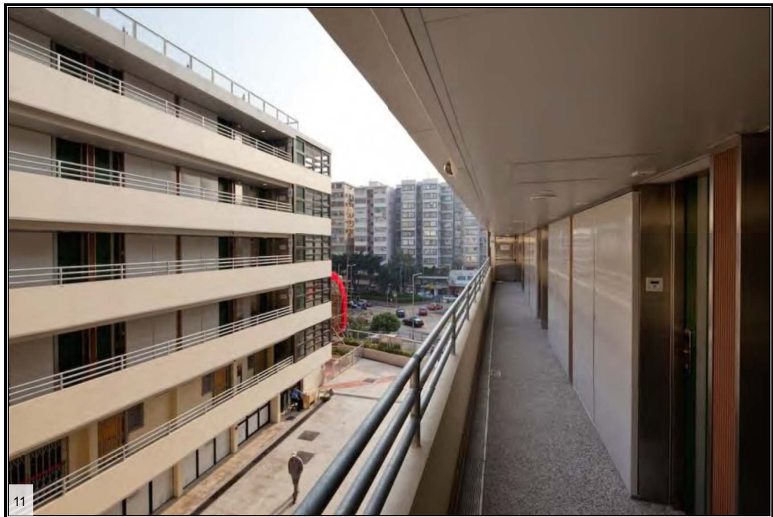
The corridor before and after the revitalisation (Source: Hong Kong Youth Hostels Association UNESCO Report (Top); AD+RG (Bottom))
