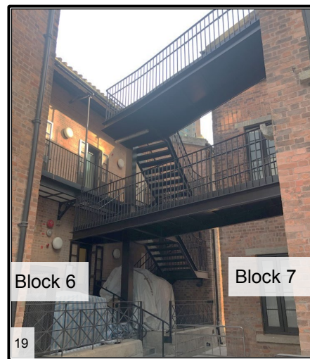
A new steel staircase added between Block 6 and Block 7 serving as an escape staircase
