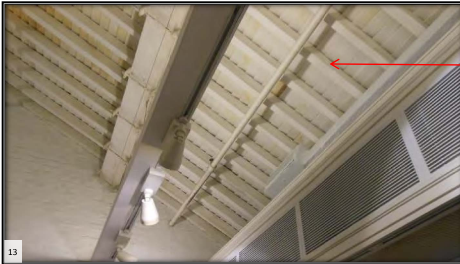
Timber pitched roof protected with fire retardant paint
