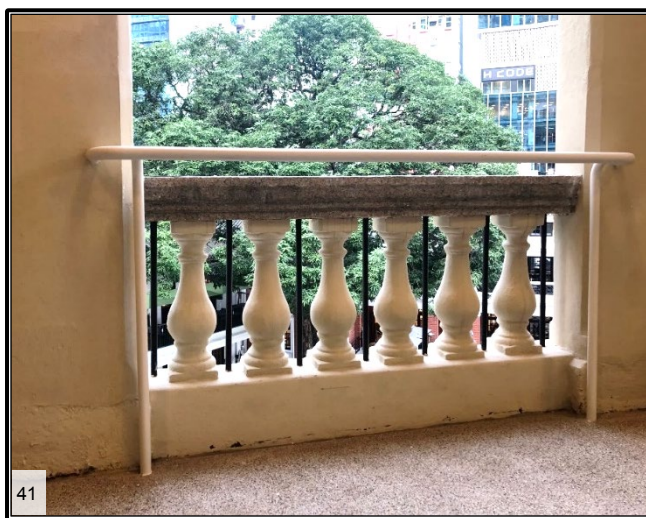
Addition of new railings and metal rods for the clay bottle balustrade of Block 3
