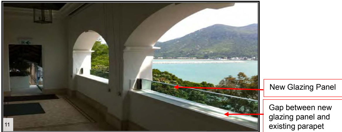
Additional glazing panels to add height to the existing parapet walls in the Main Building
