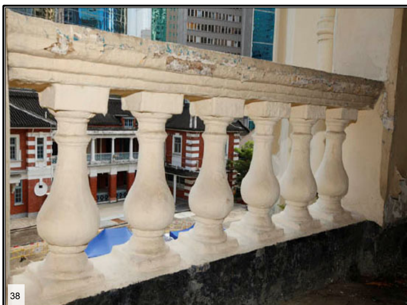
Hollowed-clay bottle balustrade before revitalisation
