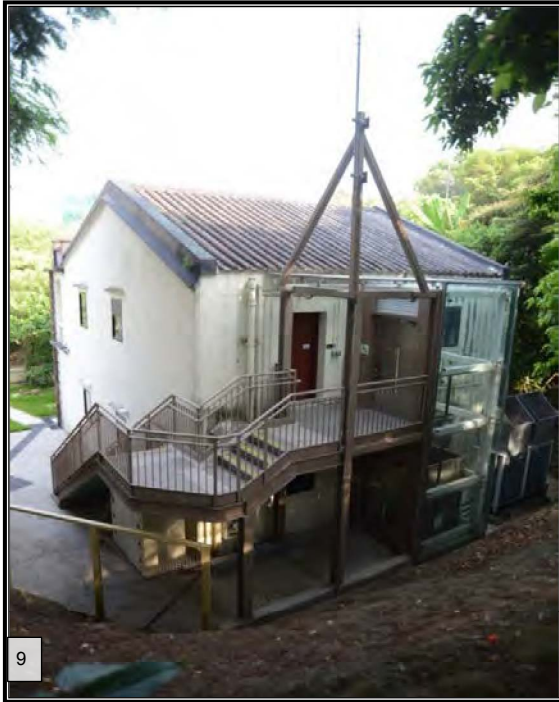
A new external metal staircase added at the side and rear elevations
