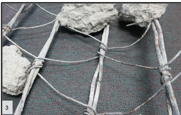
Twisted wires reinforcement revealed during open-up inspection (Source: Arup)
