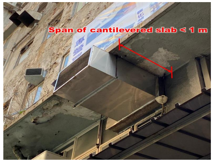
Item 2.2 Removal of ventilation duct or associated supporting frame hung underneath a cantilevered slab
