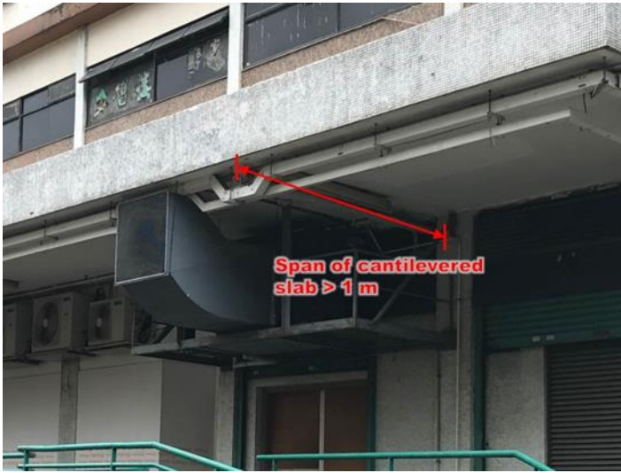
Item 1.5 Removal of ventilation duct or associated supporting frame underneath a cantilevered slab
