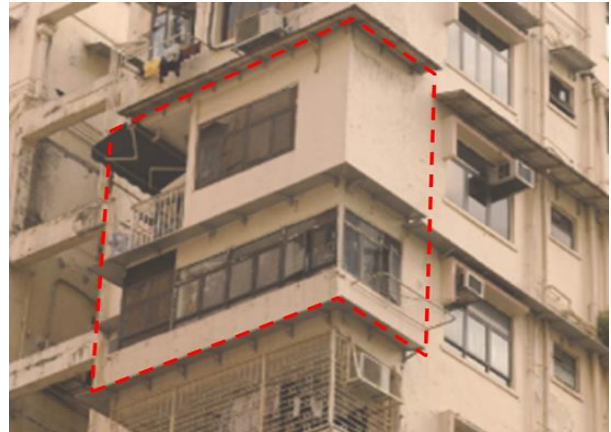
Item 2.38 Removal of unauthorised structure fixed to a balcony
