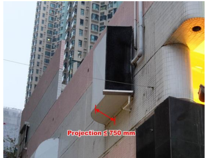
Item 3.49 Removal of ventilation duct or associated supporting frame projecting from an external wall
