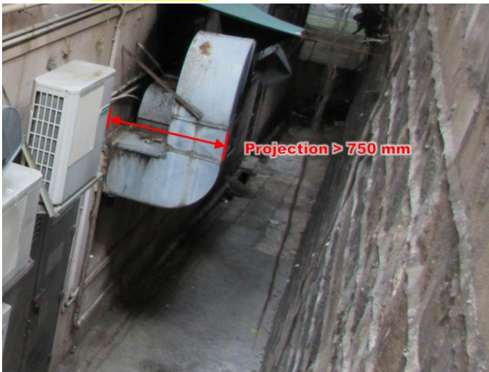
Item 2.31 Removal of ventilation duct or associated supporting frame projecting from an external wall
