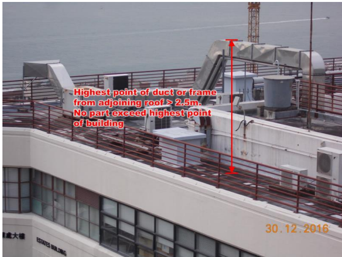
Item 1.47 Erection or alteration of external metal ventilation duct or associated supporting frame on roof
