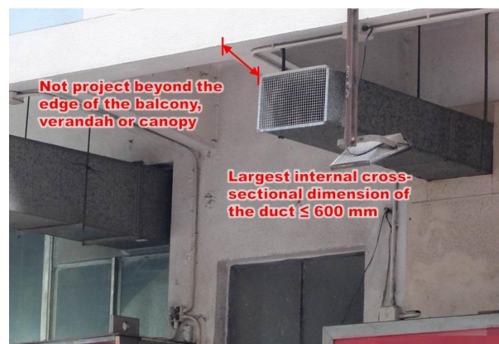
Item 3.48 Erection or alteration of external ventilation duct or associated supporting frame hung underneath the soffit of a balcony
