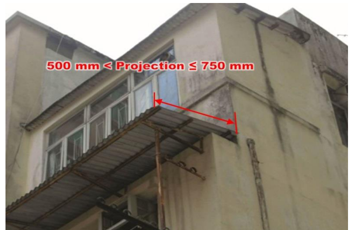
Item 3.38 Alteration of unauthorised canopy
