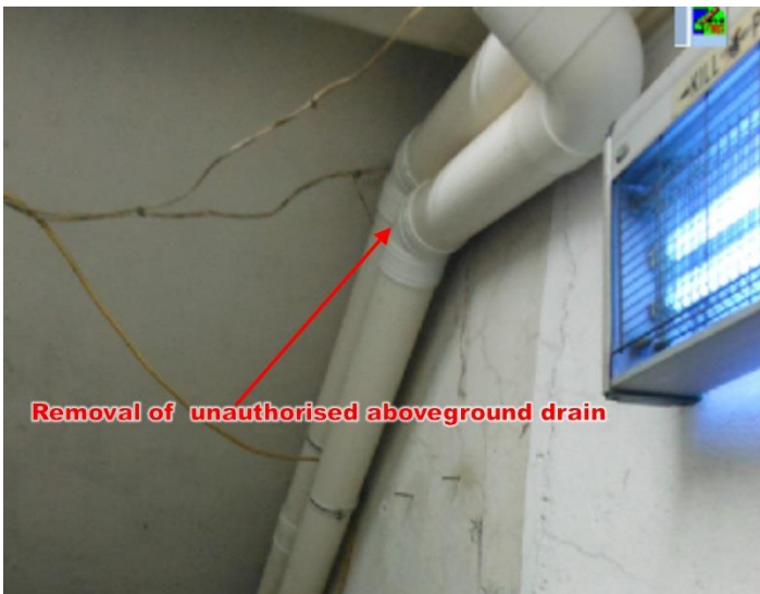
Item 3.24 Removal of unauthorised aboveground drainage
