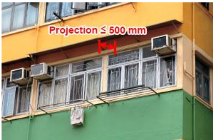
Item 3.37 Strengthening or unauthorised canopy
