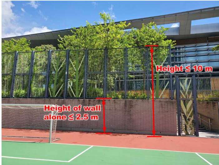
Item 1.59 Erection of mesh fence on top of solid fence wall on-grade
