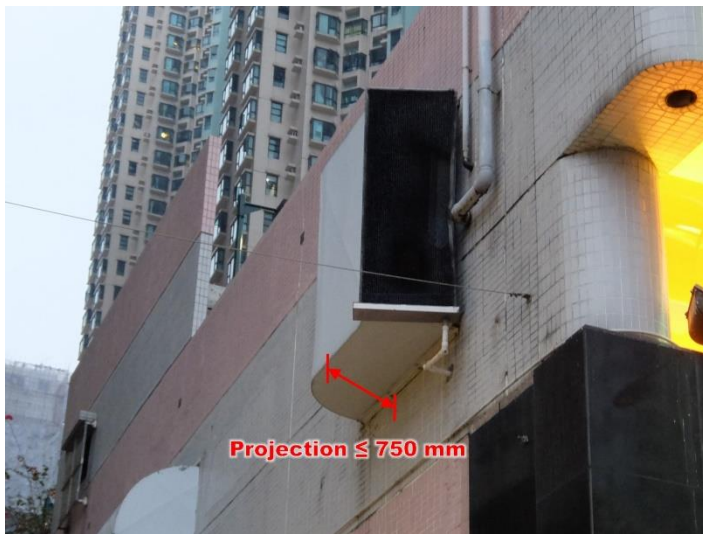
Item 1.47 Erection or alteration of external ventilation duct or associated supporting frame on external wall
