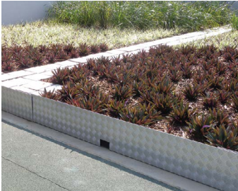
Provision of drainage outlet in greening to discharge excess water
