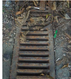
Improper maintenance of drainage system
