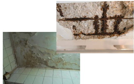
Inadequate or damaged waterproofing may result in water seepage and spalling of structural elements
